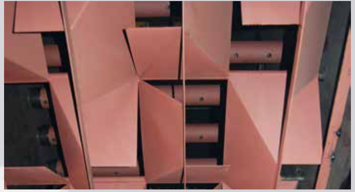
Flue gas mixer for denitrification unit
